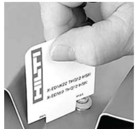
Checking the standoff of an X-EDNK22 roof deck fastening with a plastic template.
