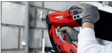
Conduits and light-duty pipes
