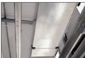
Square Air Ducts
