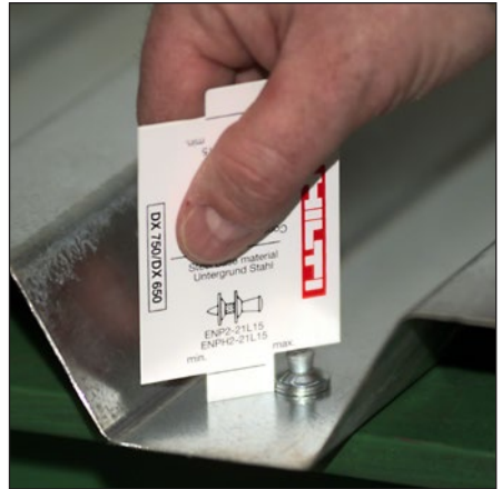
Checking the standoff of an ENP2 roof deck fastening with a plastic gauge
